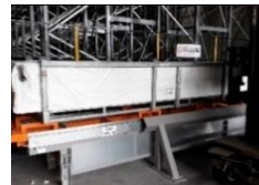
Front loading station
